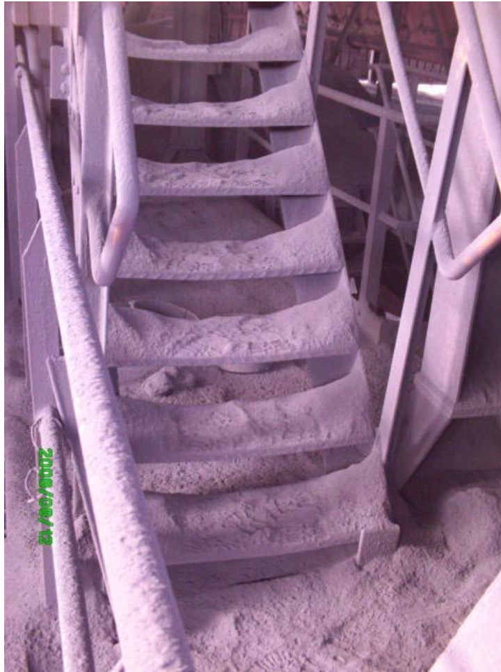
Processing Area Material Covering Stairway
