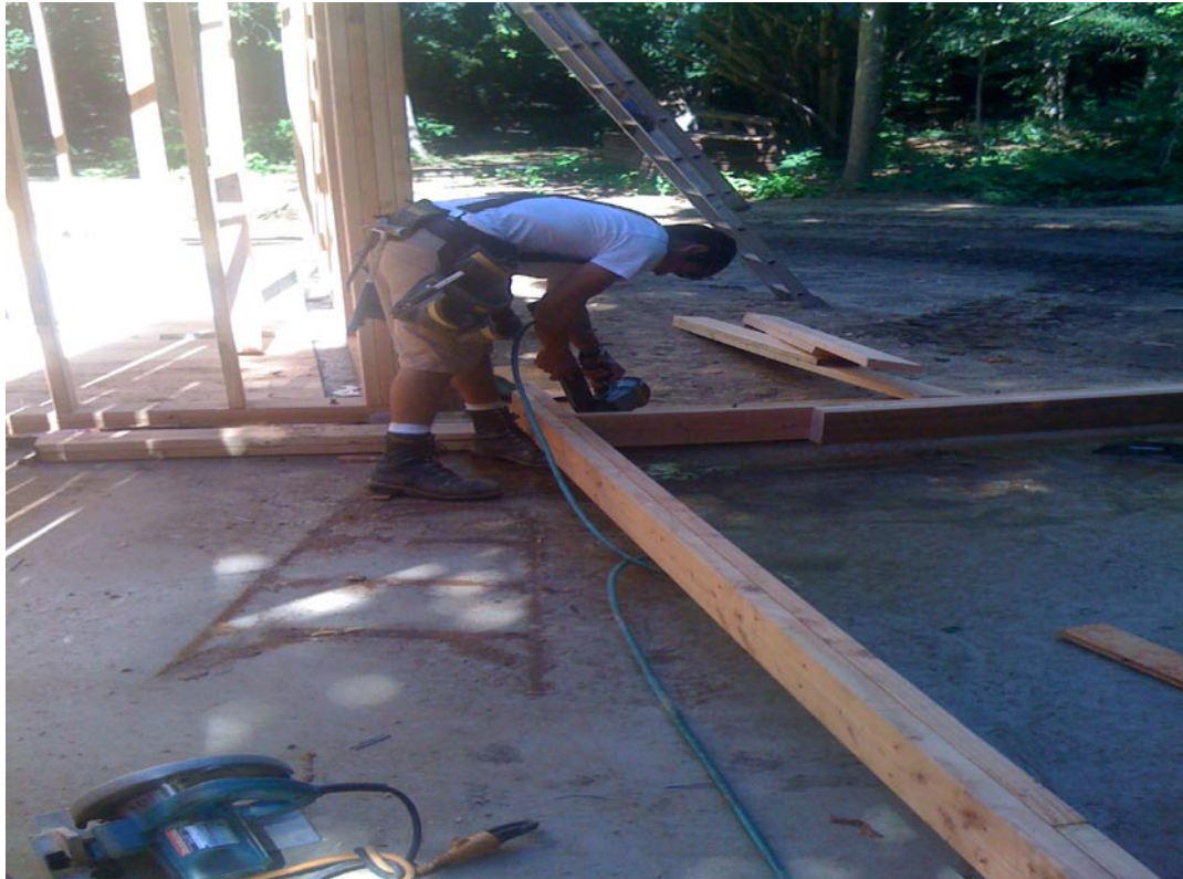
Worker not wearing safety glasses while using an air tool.
