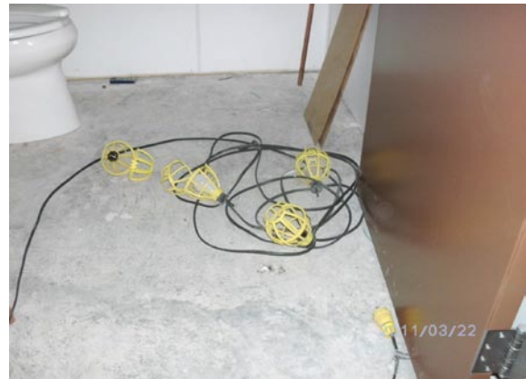
Protective light bulbs cages
